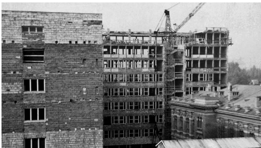
Fig. 32. The Faculty of Sanitary and Water Engineering building under construction – as it stood in October 1975
